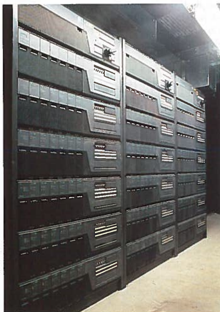
In one of the four EC90 dimmer rooms.
