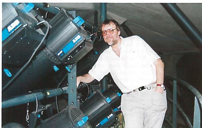
Keith Benson with ADB luminaires on the 'doughnut' walkway, high above the auditorium.
