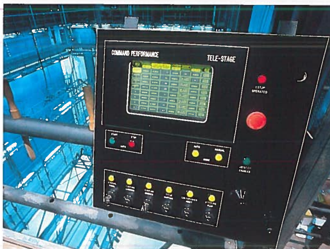
Telestage's Touchscreen computer flying control panel on the flyrail.
