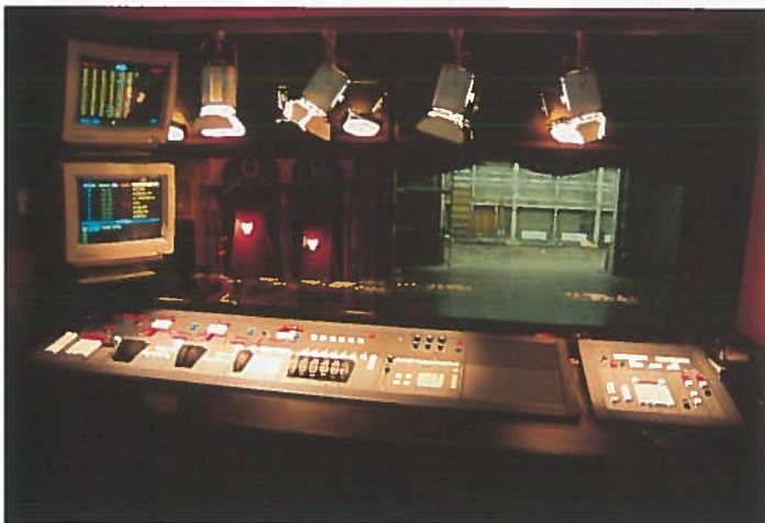
Lighting control: the Strand Galaxy Nova in the control room.
