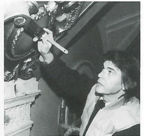
American consultant David Hannivan at work restoring the theatre to capture a look of elegance and age that would have occurred naturally had the building been maintained with its original finishes and decor since 1928.
