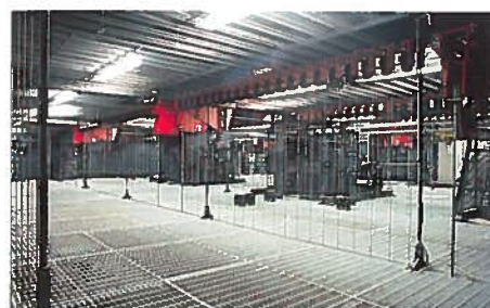
The grid with lighting bridge motors in background.
