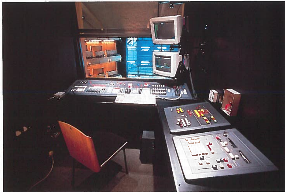
The lighting control room with a Strand Galaxy Nova.
