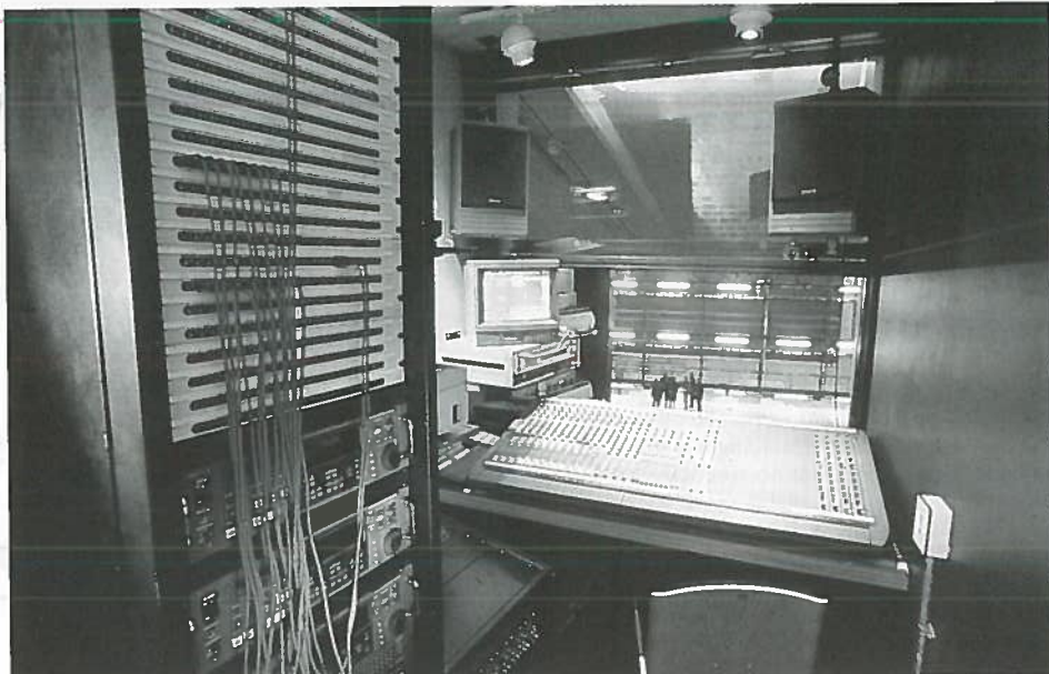
The sound control room featuring a Soundcraft Venue console.
