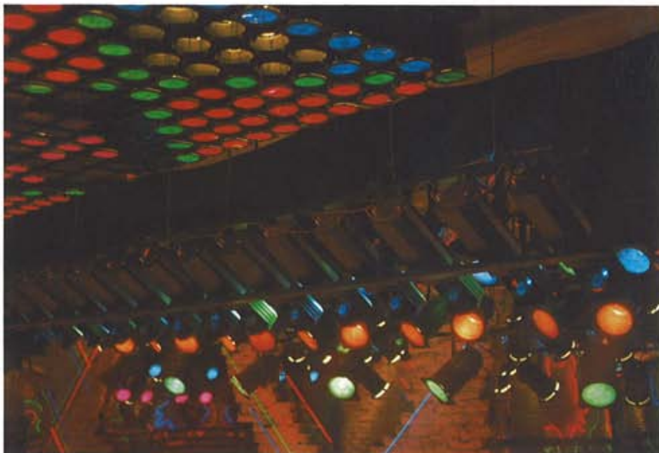
Above-stage colour, showing part of the central bank of Majorbeams, the row of 14 Coemar Robots, and a mix of Raylights.
