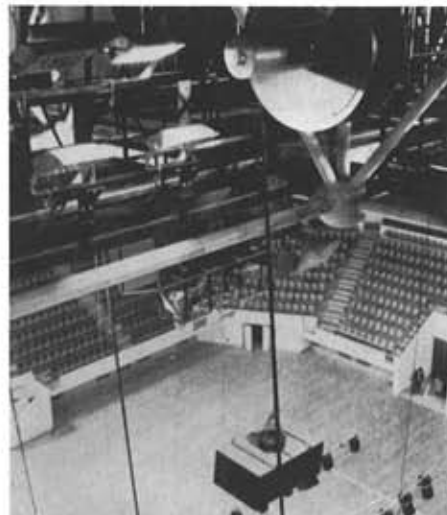
Specialist lighting and control equipment supplied and installed by Furse at the Shenzhen Coliseum, Canton, China.
