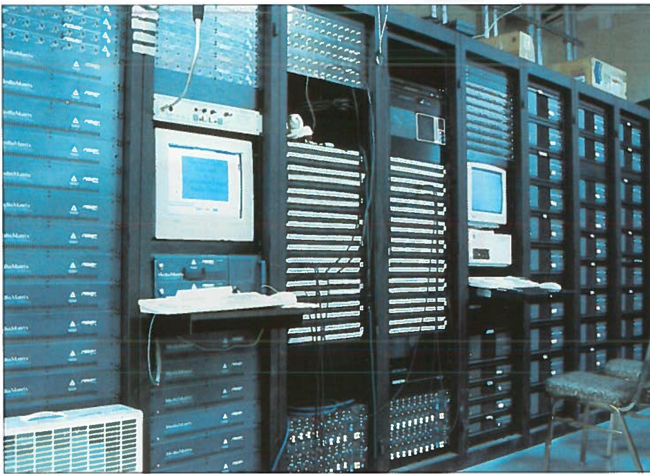
The main control room, with Peavey's MediaMatrix and the NexSys control systems side by side.
