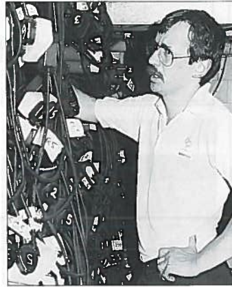
Michael Odam in the dimmer rack cage beneath the stage of the Prince Edward Theatre for 'Anything Goes' .
