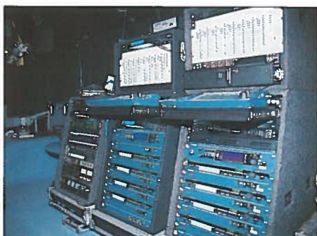
Above, the BSS/Midas XL88 loudspeaker drive racks
