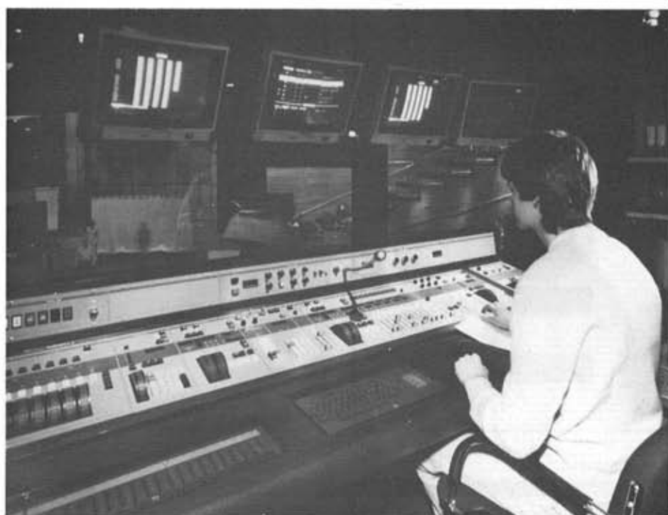
The 528 channel Strand Galaxy installed in the National's Lyttelton control room.
