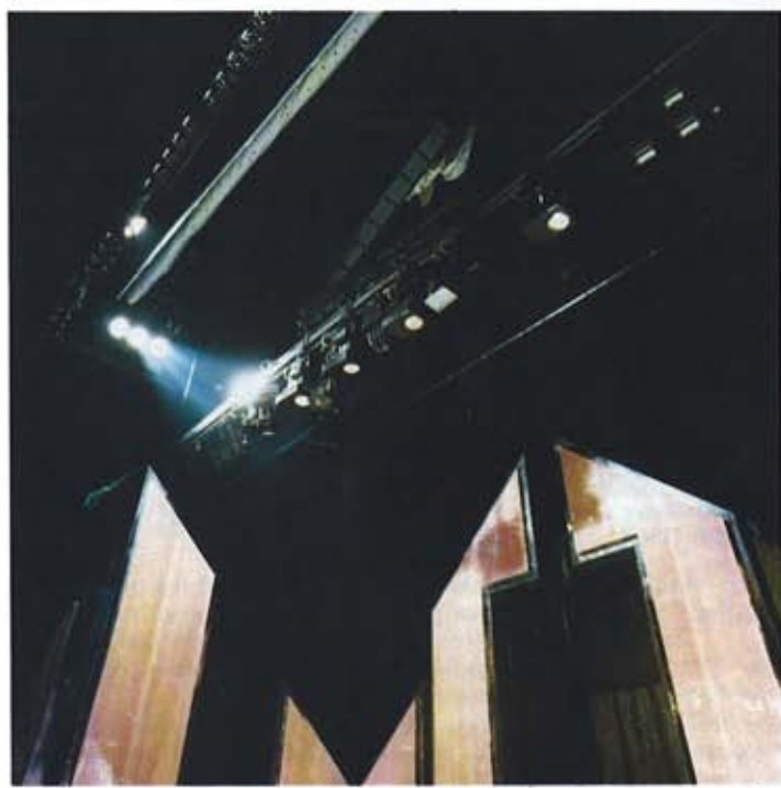
12 PEF-M motorised lighting units were installed at the Volkstheater, Vienna by Ludwig Pani in 1980.
