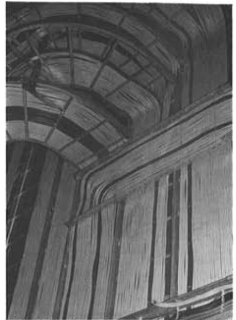
Cable-clad walls - only one 'level' of cable was allowed, on either 'ladders' or 'trays'.
