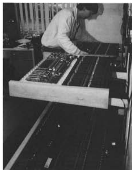
Part of the final assembly, soak testing and quality assurance area at Celco.
