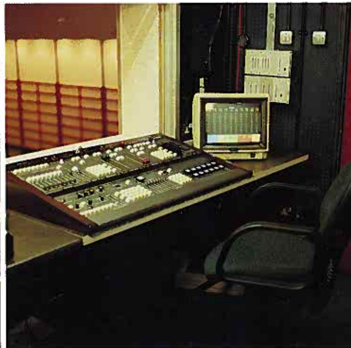
Lighting control is a 180-way Strand Gemini system.
