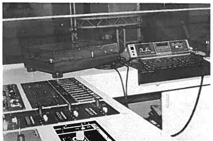
. . . and from the inside, with lighting controls to the left.
