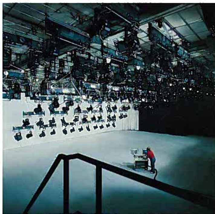
Operation of hoists and luminaires from the studio floor control.
