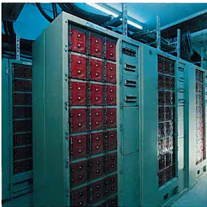
PIP dimmer racks.
