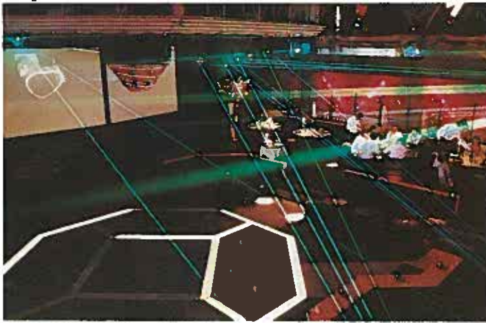
Lasers at the Casablanca Hyatt Regency were installed by SuperVision in conjunction with Laser Systems Limited.
