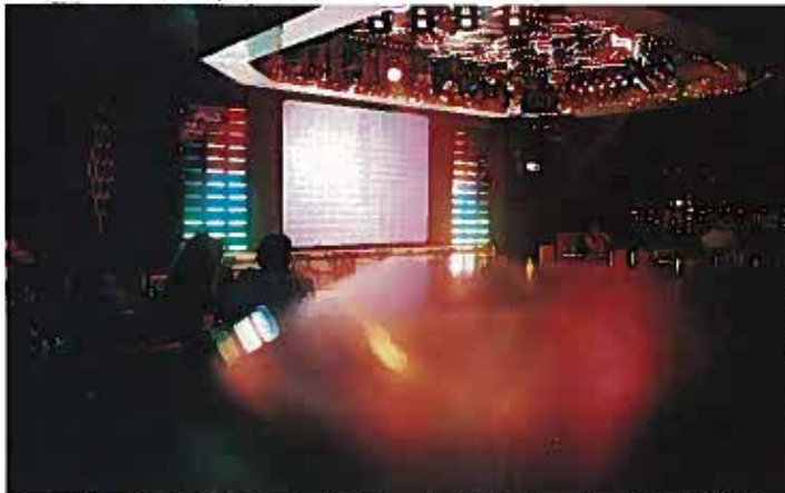
SuperVision designed, supplied and installed the complete scheme for the Heliopolis Movenpick Hotel in Cairo. The scheme features a bar graph sound-to-light display and the biggest video screen in Egypt.
