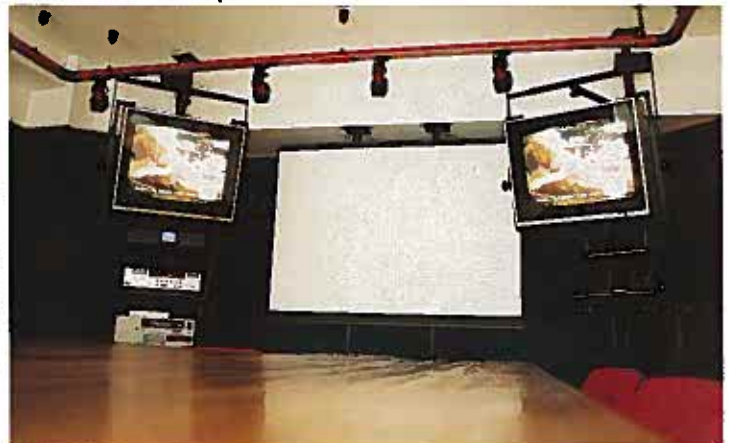
SuperVision installed this complete AV presentation scheme for a major London advertising agency in 1987. It was one of two schemes for the same client, plus a moveable system.
