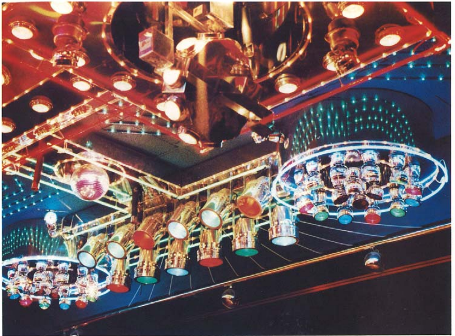
Installation at "Papillon"—Stormont Hotel, Belfast.
