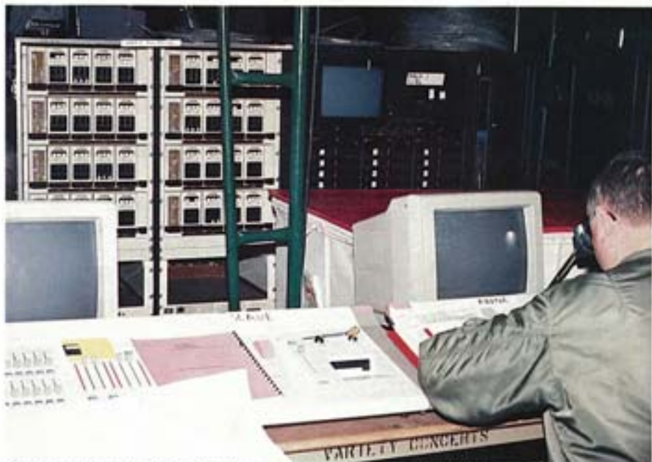
Lighting control centre for the 31st Grammy Awards, backstage at The Shrine.
