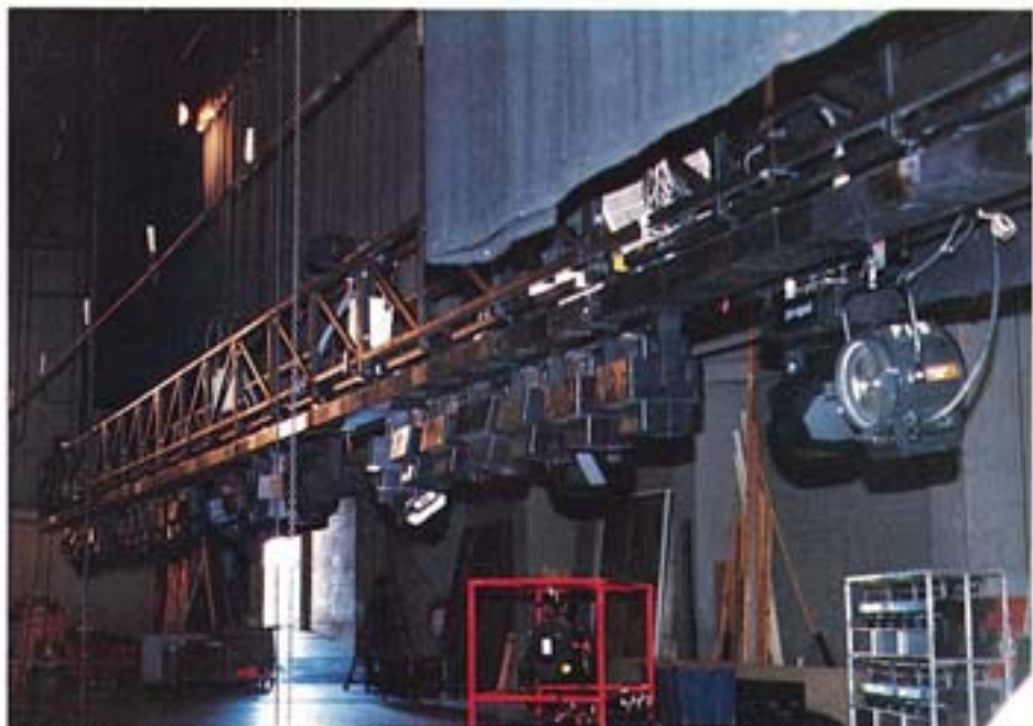
Set-up at The Shrine: one of the huge multi-section Morpheus Flip Box Truss systems ready for flying, the protective 'cage' having been lifted up to form the catwalk above.
