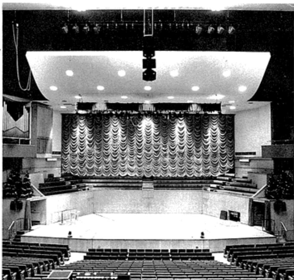
The Meyer loudspeaker cluster at Croydon's Fairfield Halls was installed by Wigwam.
