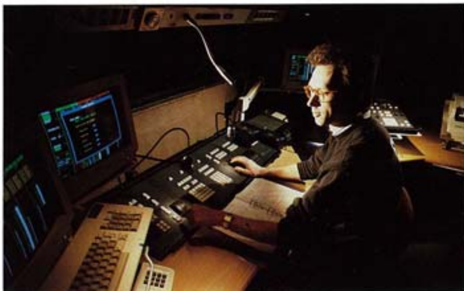
The ADB lighting control installation, Gothenburg City Theatre.
