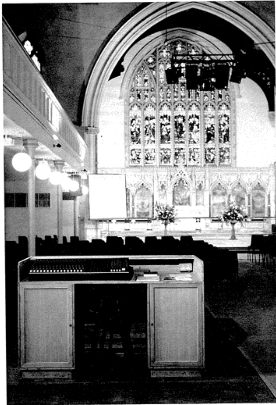
The sound system at St. Paul's Church, Onslow Square, London was installed by Wigwam Contracting.
