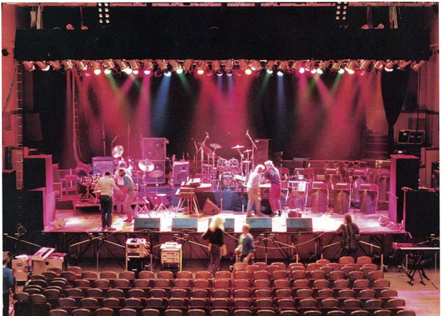
The new look lighting and sound rig installed at Wolverhampton Civic Hall.
