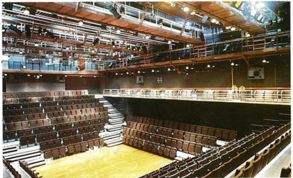
The Studio Theatre with over 160 Strand luminaires installed.
