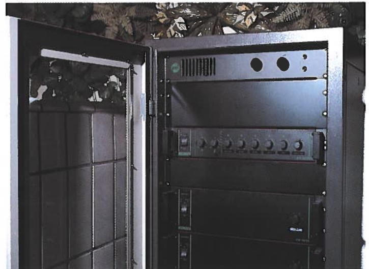
Control rack in the Water World complex.
