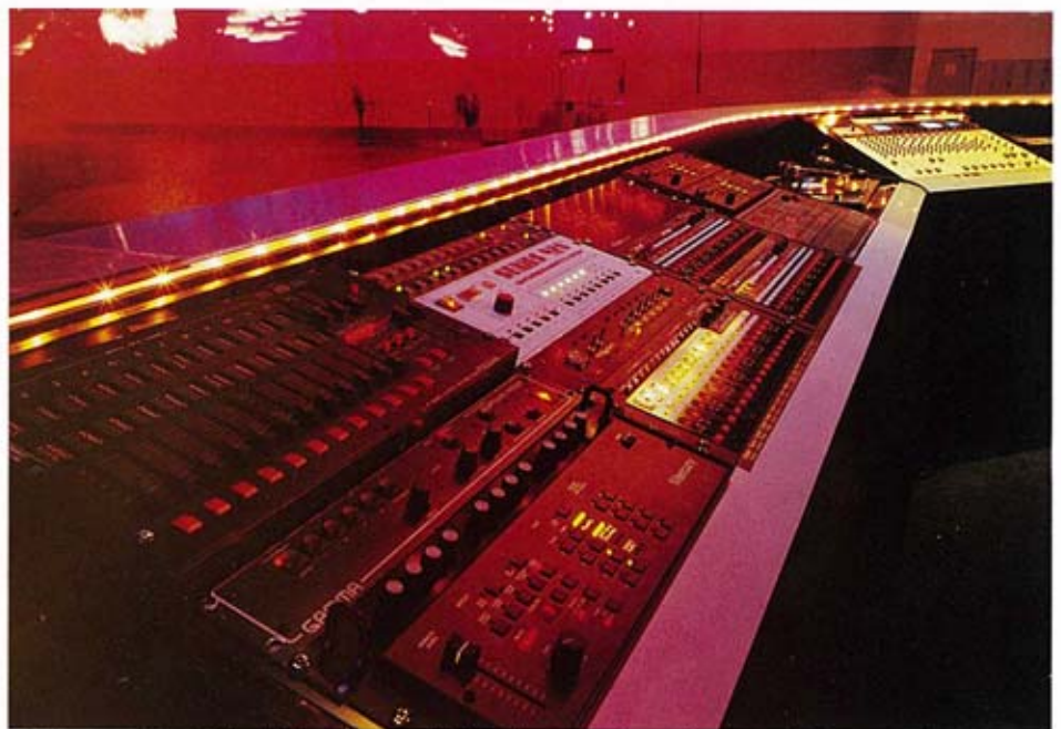
On the operational side, Avitec have specified Mode 16 touch panels to control the massive lighting rig.
