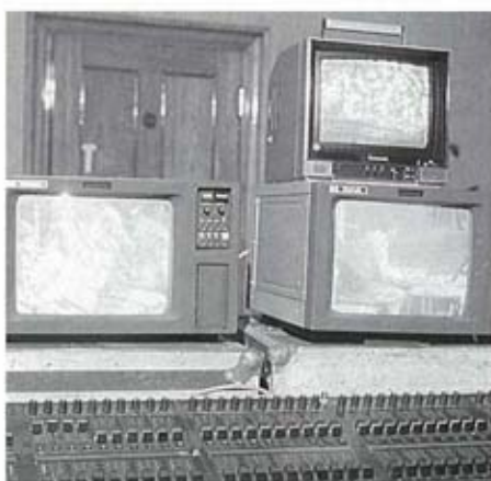
Control is courtesy of two Celco's running through the Q-Patch system.
