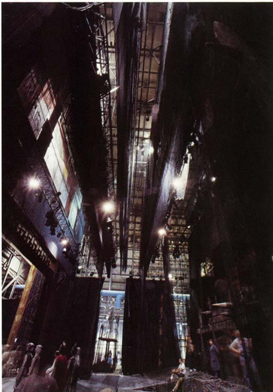
View from stage left counterweight side with bars being loaded.
