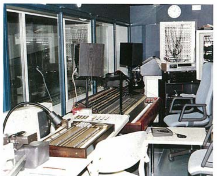
The small auditorium control room.
