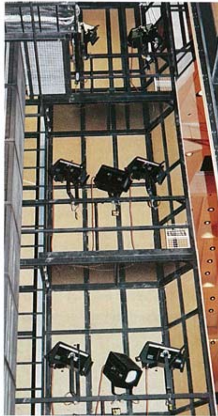
Lighting positions, side stage.
