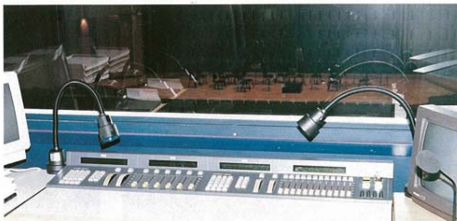
The Helvor Macro II in the Concert Hall lighting control room.
