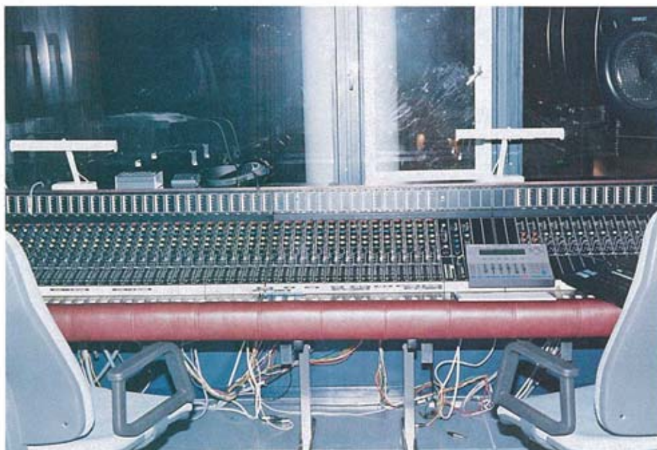
MS-Audiotron MCA Multimix system at Tampere Hall.
