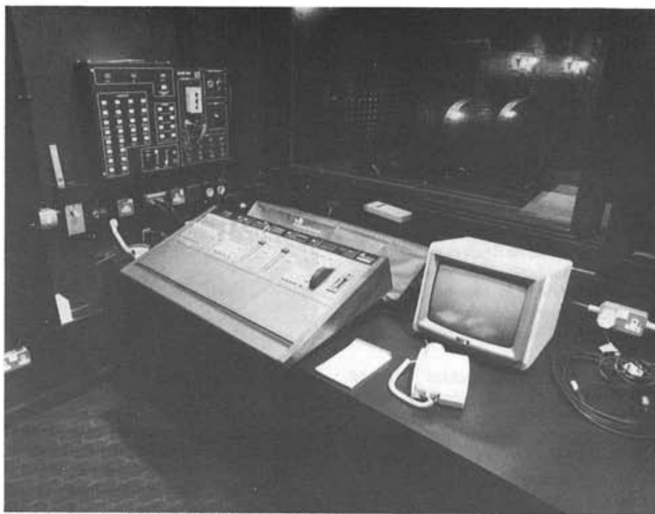
Control room showing Gemini lighting control board.
