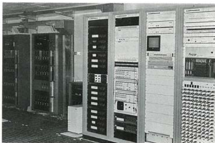
One of the four dimmer rooms situated in the I Corsari complex.
