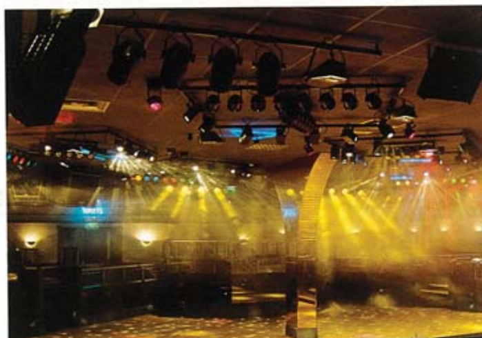
Specialist effects lighting for the Middleton Park Hotel, County Cork.
