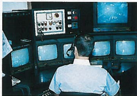
The main control centre.
